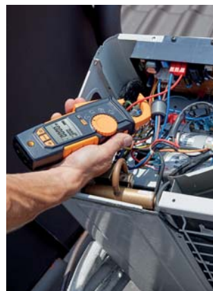
Measuring the current by clamp meter in outdoor unit of air conditioner.
