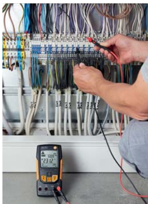
Testing voltage in a switching cabinet.
