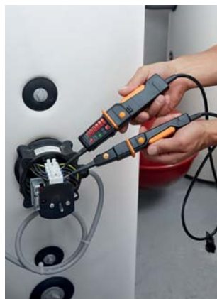
Measuring voltage on a boiler.
