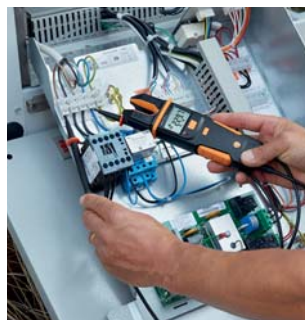
Measuring voltage on a compressor.
