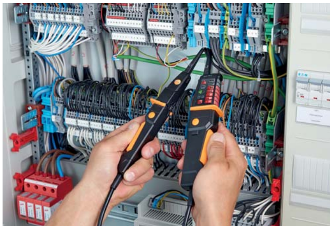
Measuring voltage in a switching cabinet.
