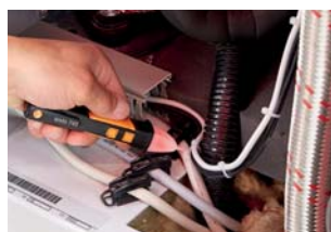
First test of voltage supply on a compressor.
