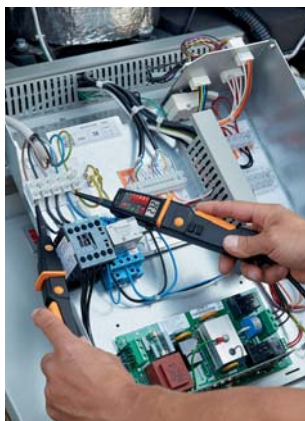
Measuring voltage on a compressor.
