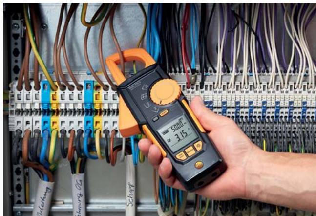
Measuring current in a switching cabinet.
